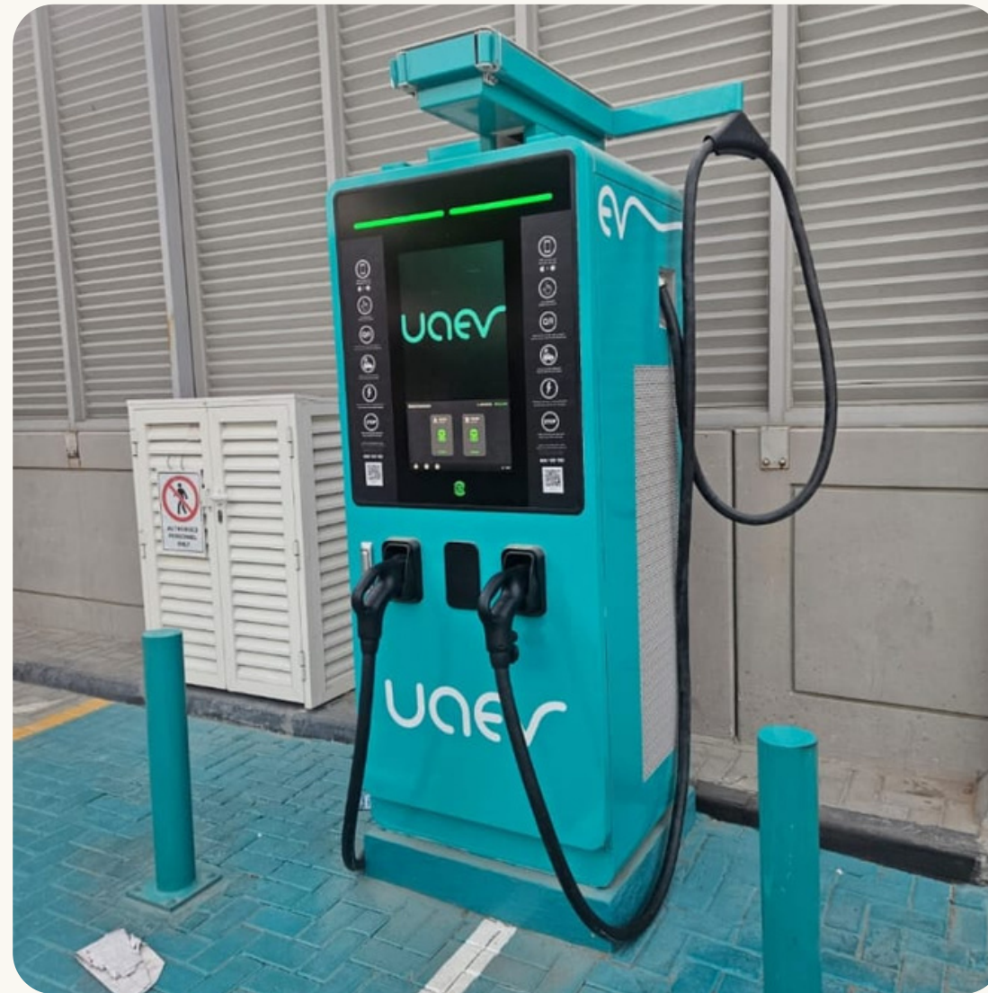
200 KW charger at EMARAT PETROL STATIONS
