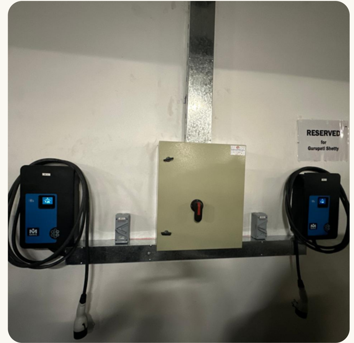
22 KW charger at FORD In Sheikh Zayed Road
