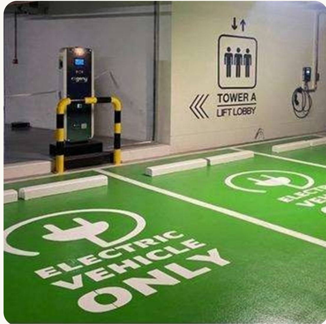
Multiple 44 KW chargers at OPUS by OMNIYAT
