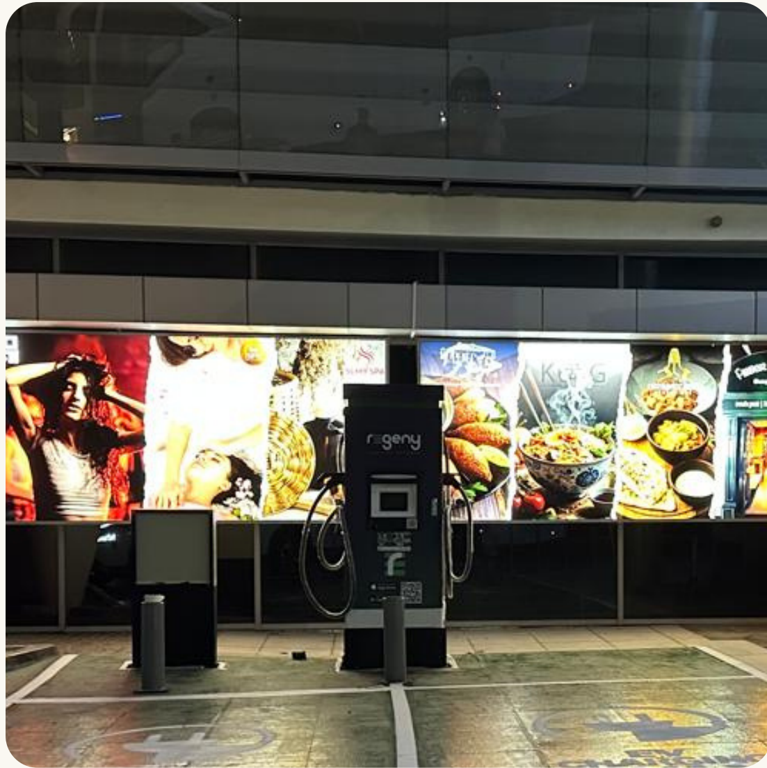
120 KW charger at SOCIAL HOTEL AL BARSHA
