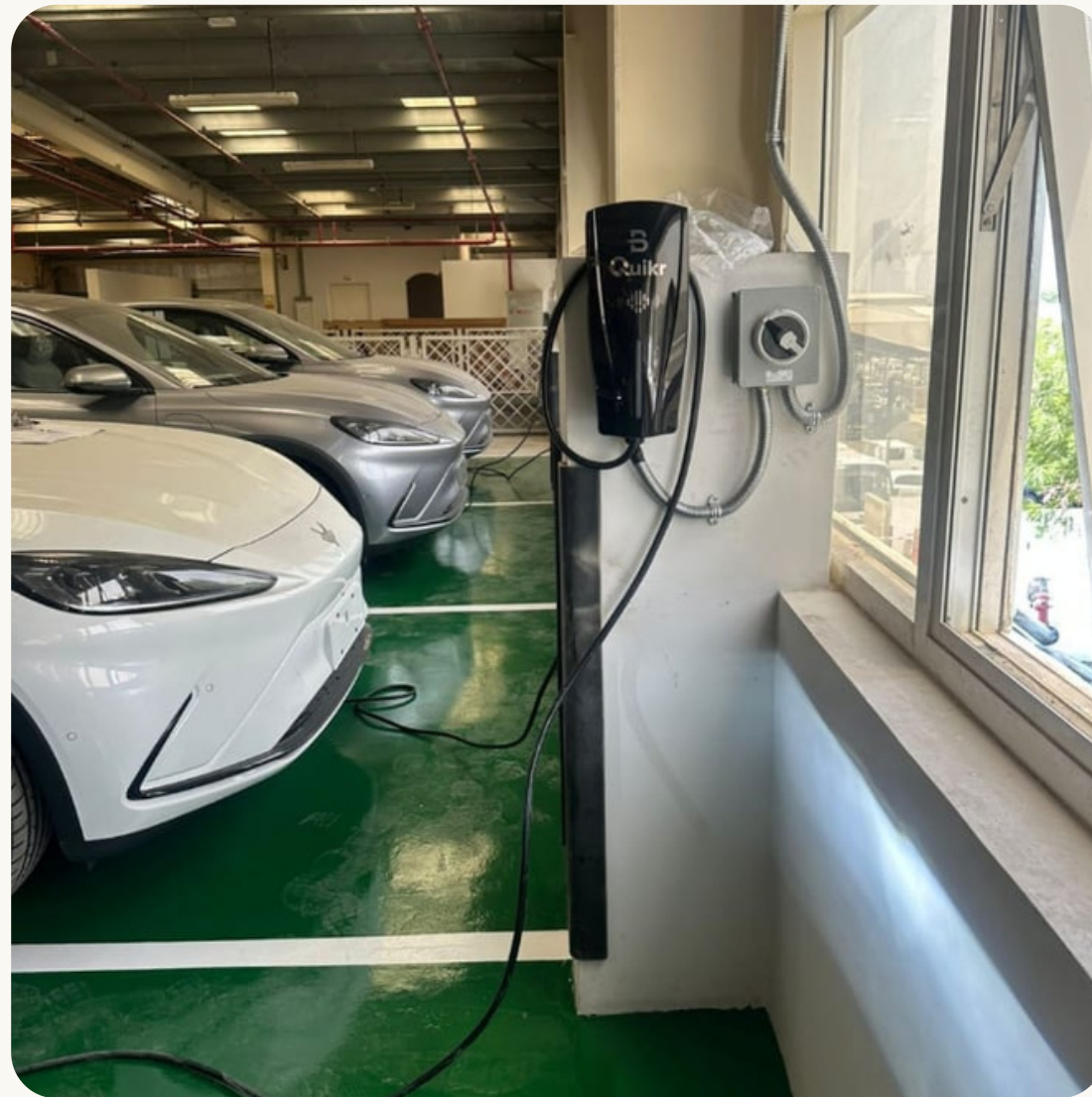
22 KW charger at SUBARU WAREHOUSE
