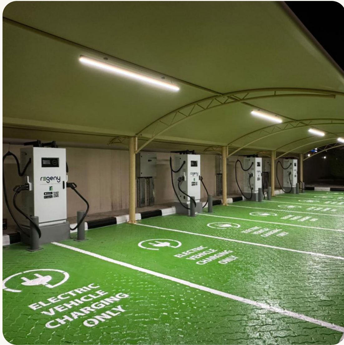
150 KW chargers at MOVENPICK AL BUSTAN
