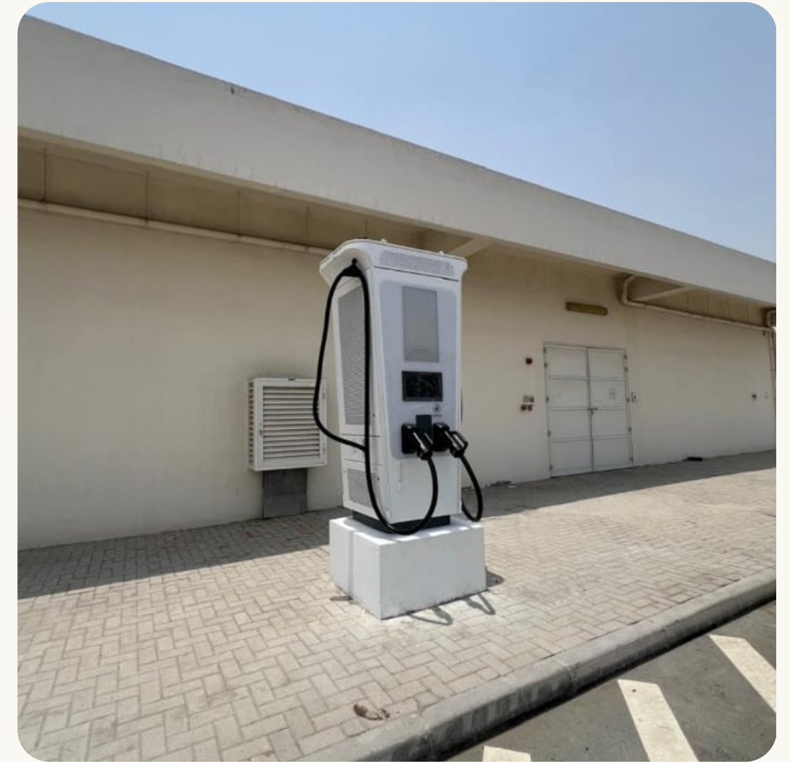
360 KW charger at RTA RUWYYAH BUS DEPOT
