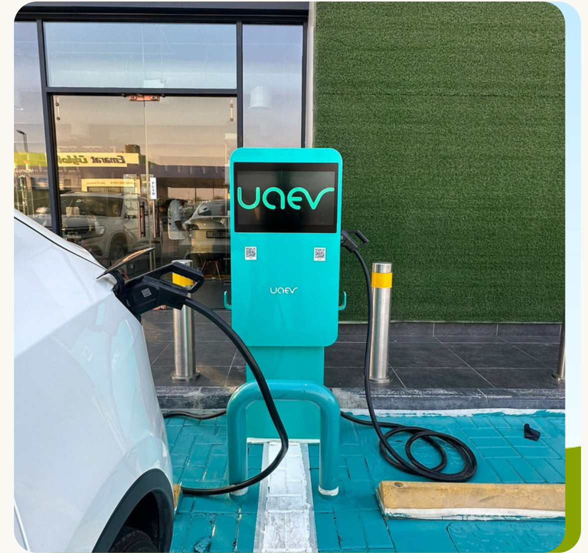
50 KW charger at EMARAT PETROL STATIONS
