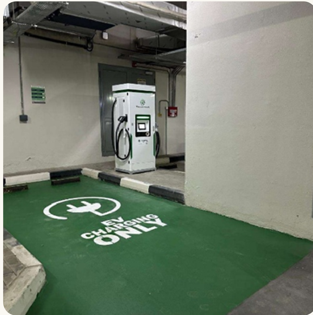
60 KW charger at LAMAR MALL
